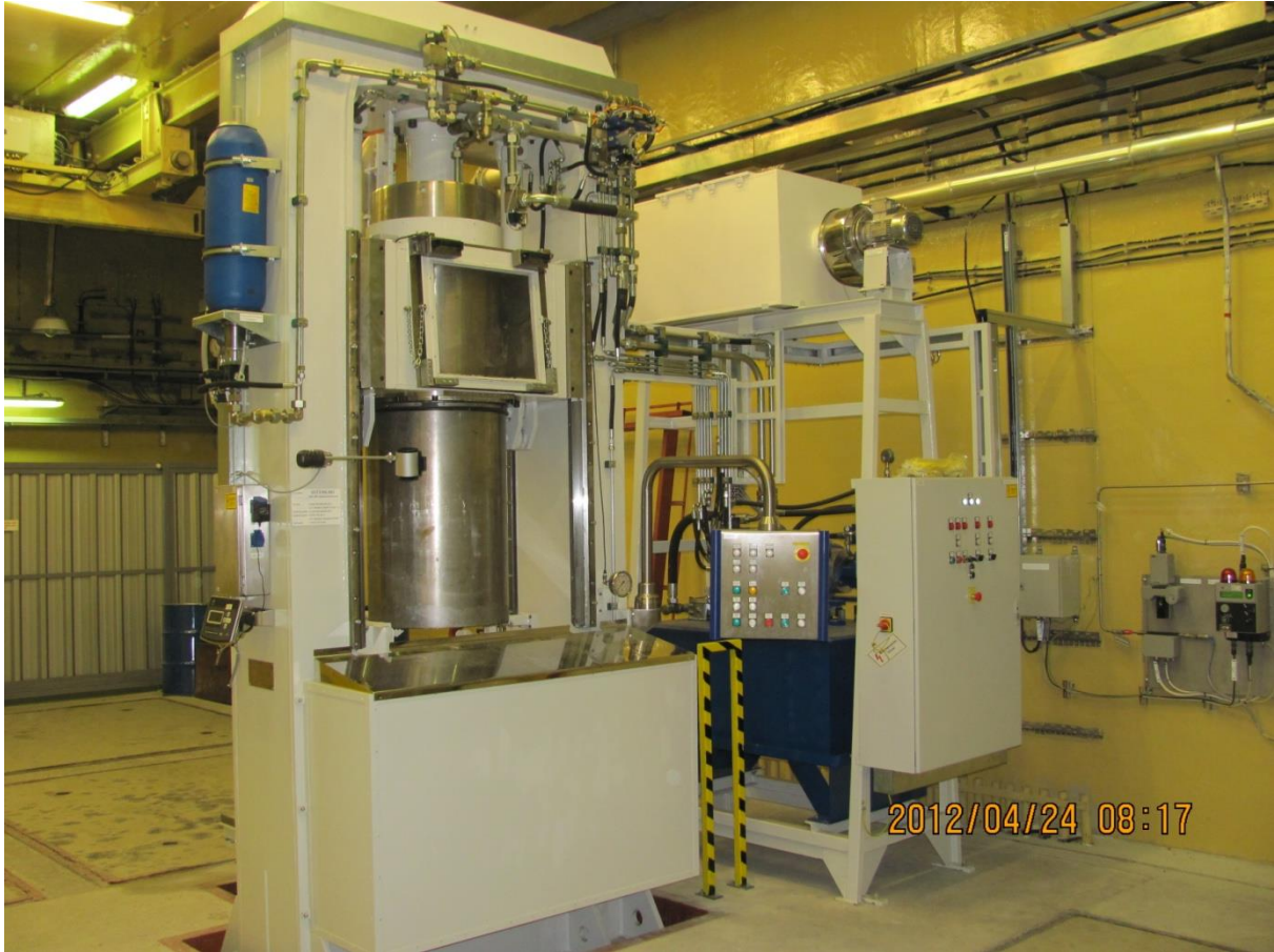
Figure D.2.4 – 2. Waste compressor machine
